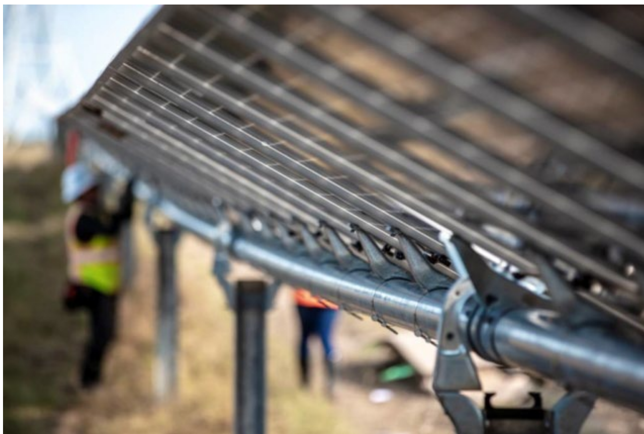
Photo 1.2 Example of Typical Single Axis Tracking System
