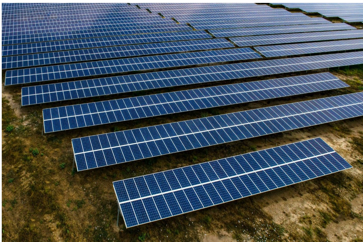
Photo 3.1 Example of Solar Panels (Umwelt, 2021)
