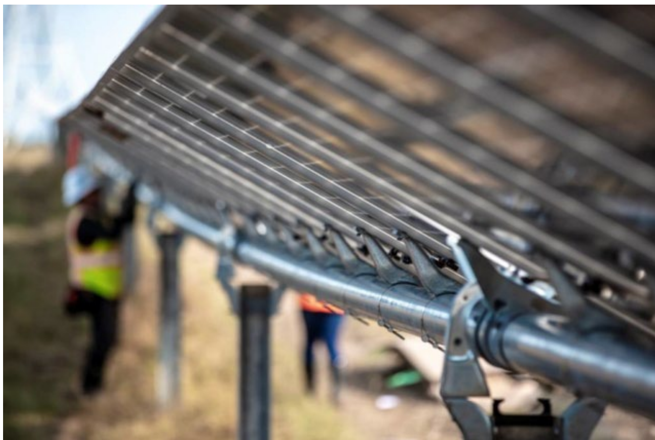
Photo 3.2 Example of Typical Single Axis Tracking System
