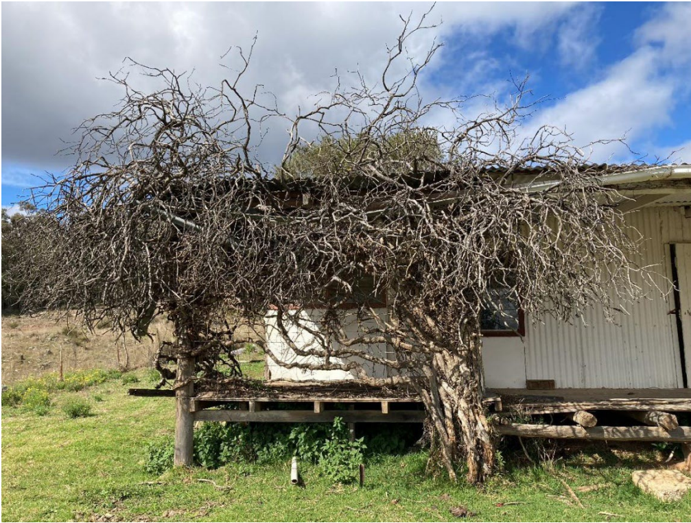
Photo 4.5 Prominent plant growth dominating the front façade of the dwelling (1900 house)
