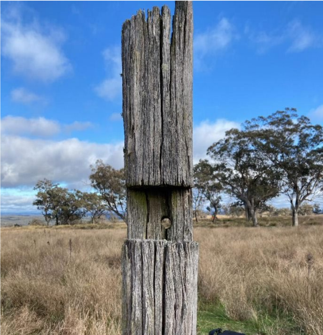
Photo 4.16 Evidence in joinery work (Slab Hut)
