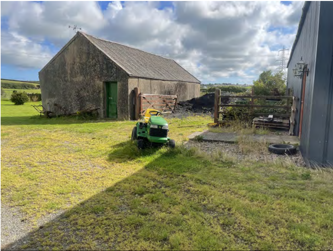
Photo 5—Farm buildings adjacent to fields east of Llyn Alaw. Possible asbestos containing materials within building fabric.
