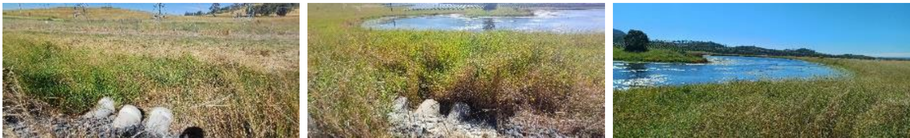
Plate 9 Culvert 9 WWBW conditions. Left to right showing culvert facing south; culvert facing north; and general condition of the waterway.
