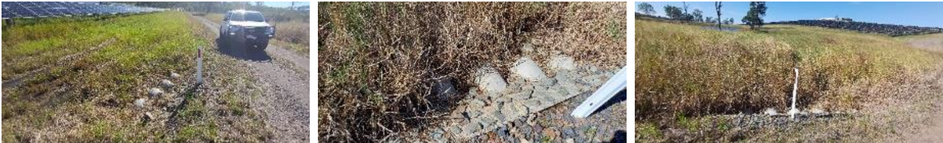
Plate 6 Culvert 6 WWBW conditions. Left to right showing culvert facing southwest; culvert facing north; and general condition of the waterway.
