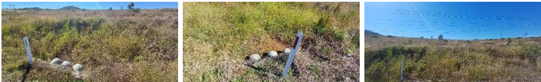
Plate 8 Culvert 8 WWBW conditions. Left to right showing culvert facing northeast; culvert facing south; and general condition of the waterway.
