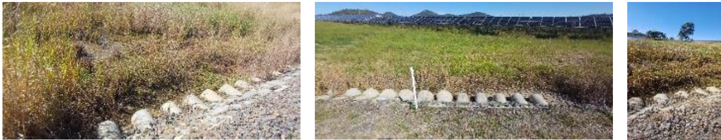
Plate 7 Culvert 7 WWBW conditions. Left to right showing culvert facing north; culvert facing south; and general condition of the waterway.
