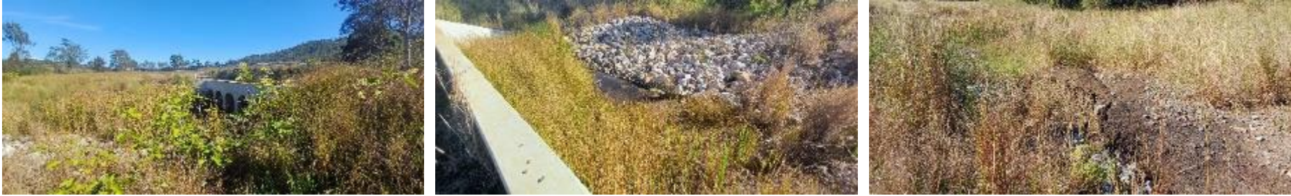
Plate 4 Culvert 4 WWBW conditions. Left to right showing culvert facing south; culvert facing north; and general condition of the waterway (washdown on bank).
