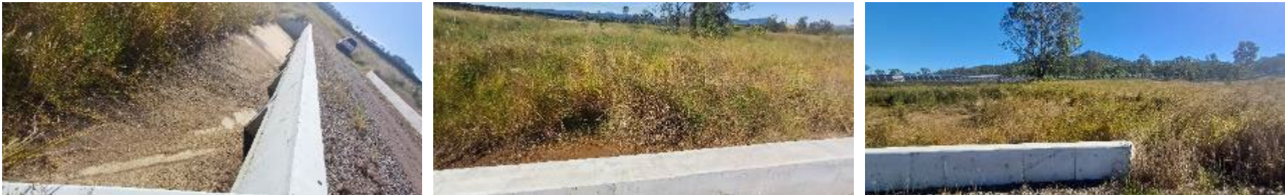
Plate 5 Culvert 5 WWBW conditions. Left to right showing culvert facing south; culvert facing north; and general condition of the waterway.
