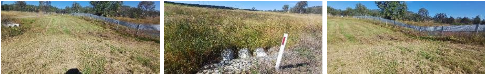
Plate 10 Culvert 10 WWBW conditions. Left to right showing culvert facing west; culvert facing northeast; and general condition of the waterway.
