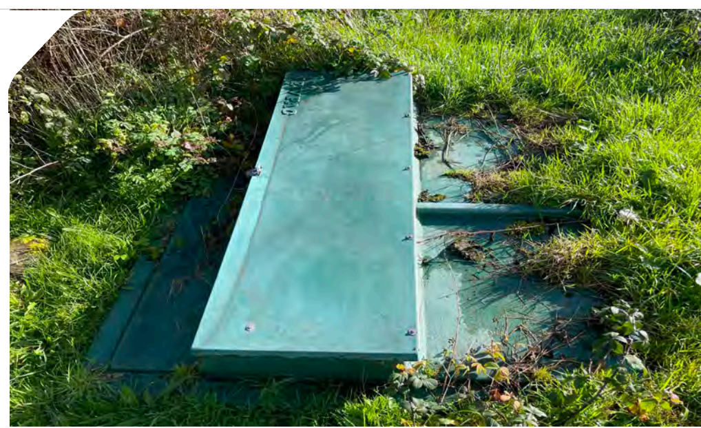
Plate 02: Field 7 – Underground Pumping Tank
