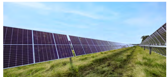
Solar panels are mounted on posts, enabling growth of vegetation underneath that allows for natural drainage and the interception of storm water
