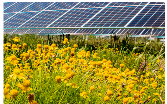
Rich ecosystem under and around solar panels shown at Lightsource bp solar farm in Texas
